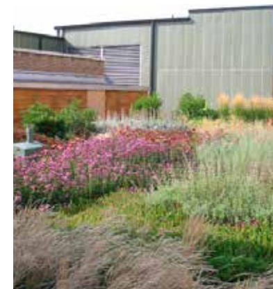
FIGURE 2.15 Native perennial planting on the Allegheny County Office building's Green Roof provide visitors with an unexpected garden.
