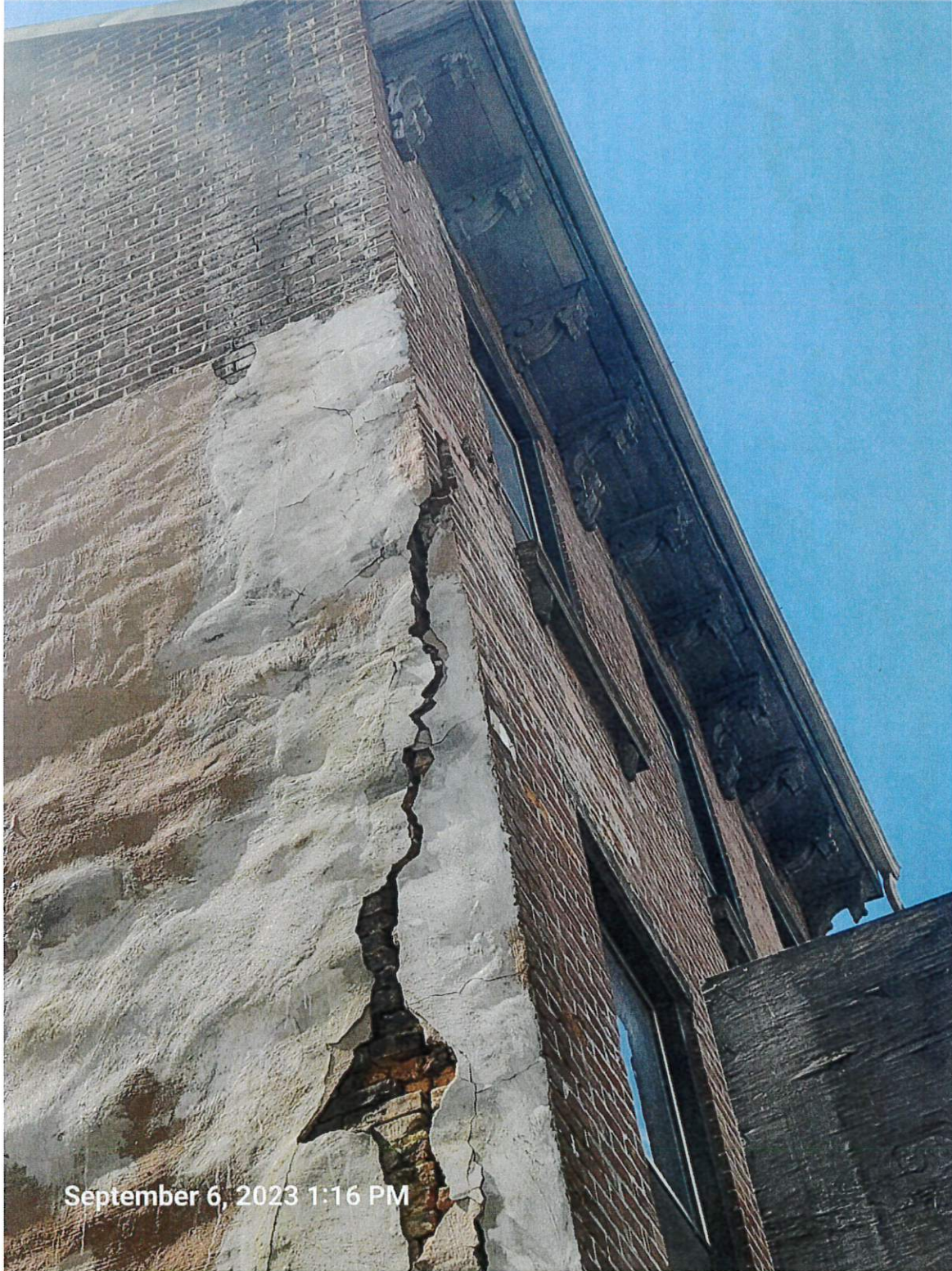
Cracking and falling debris from the left side of Subject Property if you are facing property from Fifth Avenue. Image shows how lower portion of façade is shifting away from the building towards Fifth Avenue.
